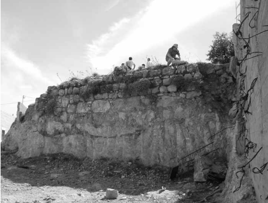
Figure 18. The north wall of the cistern on the summit of Khirbet es-Sauma'a, showing recent damage cause by modern construction. Photograph: S. Gibson.
